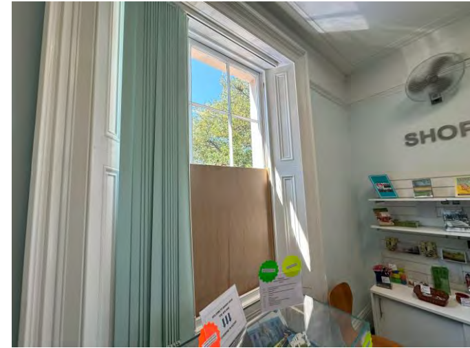
Museum Reception (002) – Sash window over-boarded
