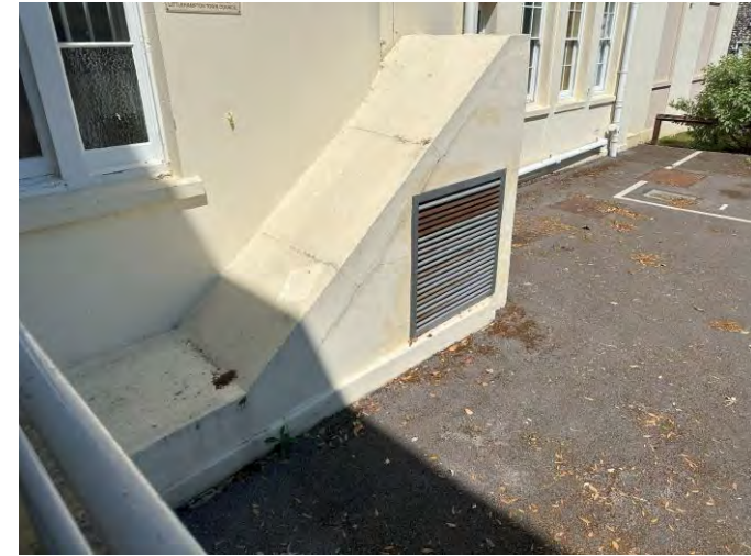
Cracking observed to boiler room fire escape
