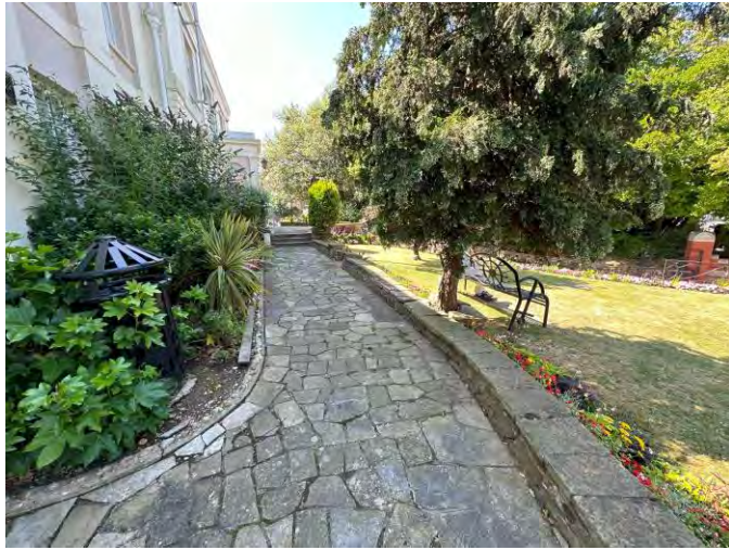
Undulations to concrete paved pathway
