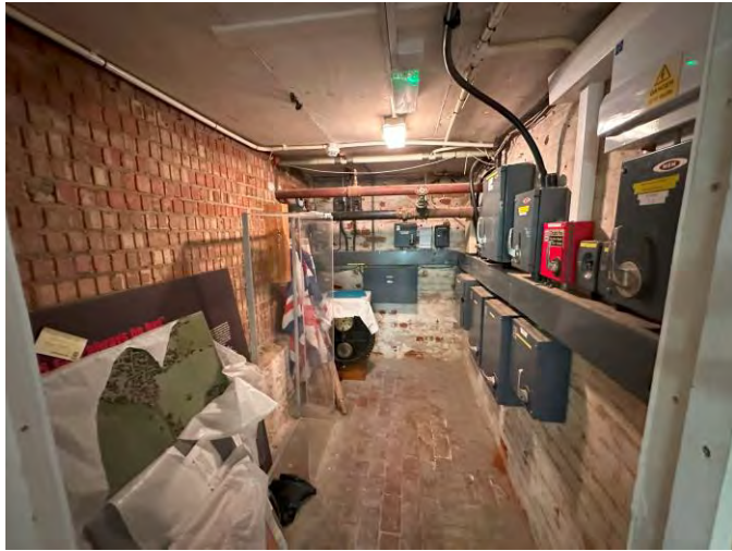
Basement – Electrical Switch Room
