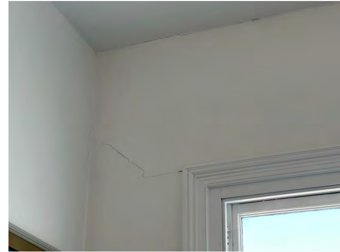
Cracking to LHS of lobby window to New Millenium Chamber
