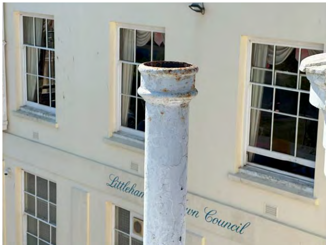
Sport corrosion to SVP
