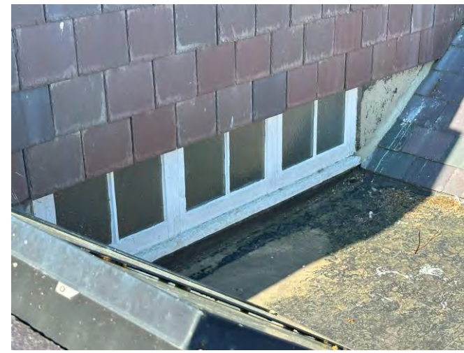
Tile hanging and timber borrowed light above stair landing – water ingress noted internally.
