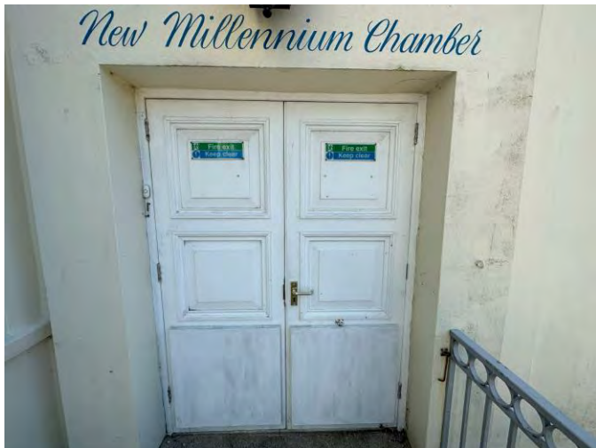
Timber framed panelled doors; painted. Bottom panels have been damaged and subsequently boarded over.
