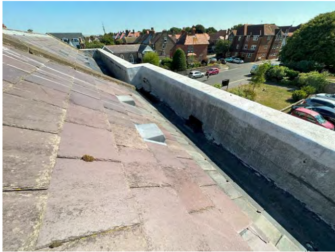
Tiled roof, roof vents and liquid applied waterproof coating / repairs to back gutters behind parapet walls
