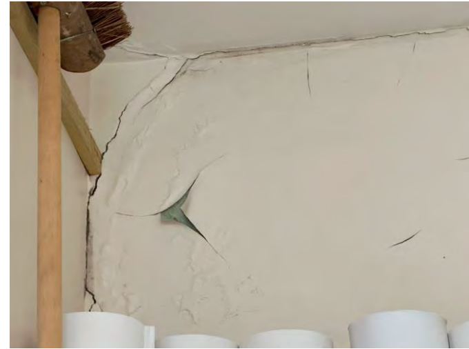
Male WC (110) Cleaners C/b – Cracking and blistered paintwork to external wall.
