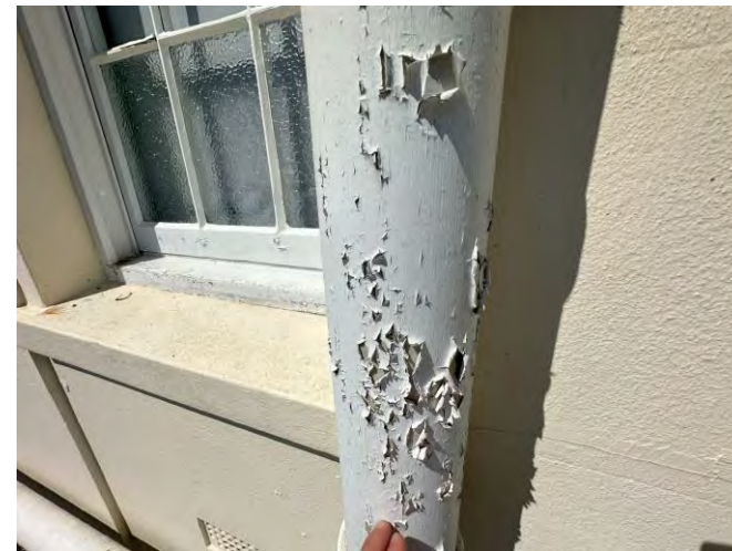
Flaking paintwork to uPVC SVP
