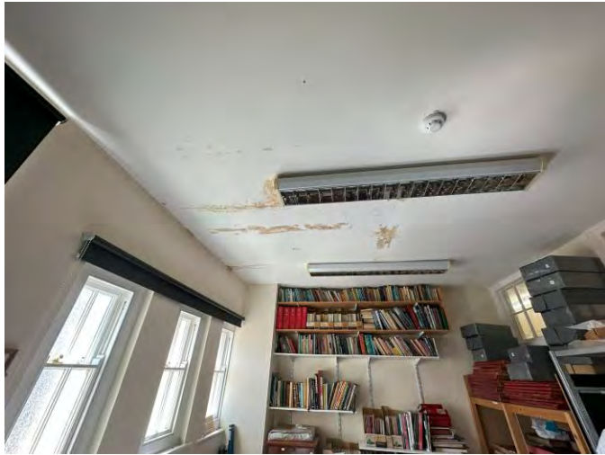
Local Studies / Stanford Office (029) – Cracking, staining and historic repairs observed to ceiling.
