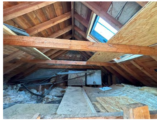
Roof void; conservation style roof lights / access onto inverted roof / mansard to adjacent parapet.
