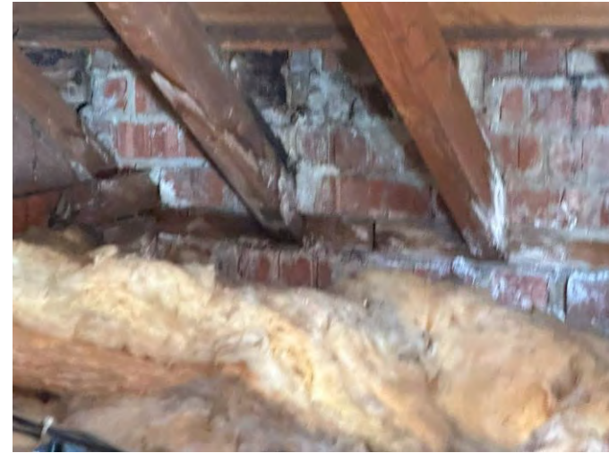
Condensation and decay observed to bottom of rafters adjacent to back gutters
