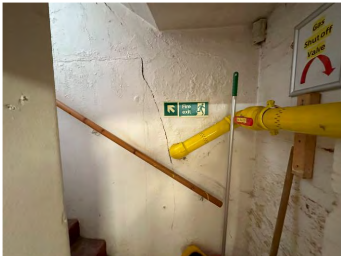
Boiler Room Staircase – Cracking observed to rear masonry wall.
