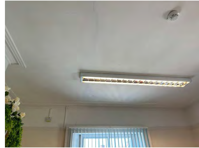
Office (114) – Crazed cracking to lath and plaster ceiling with historic damp staining observed.
