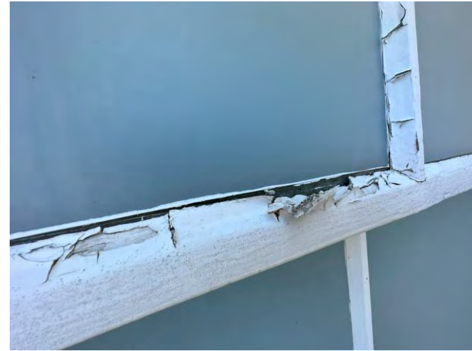
Flaking paintwork and friable putties
