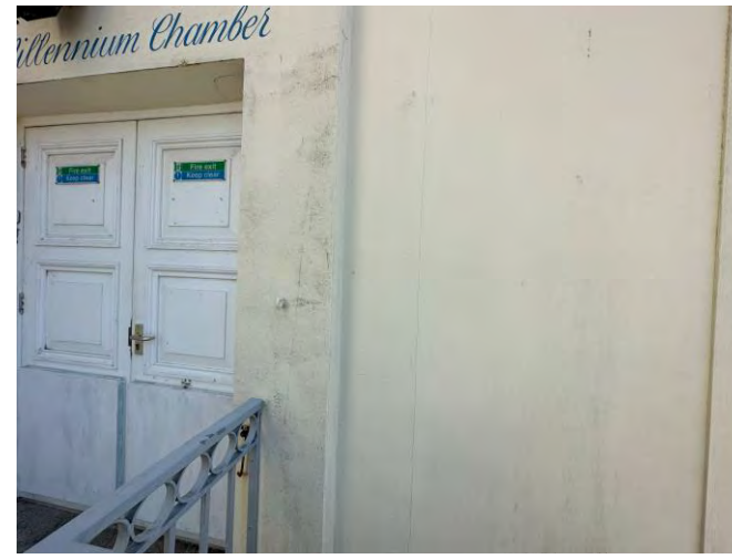
Vertical cracking RHS of New Millennium Chamber doors
