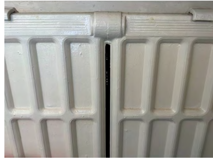
Store (118) – Daylight observed behind radiator
