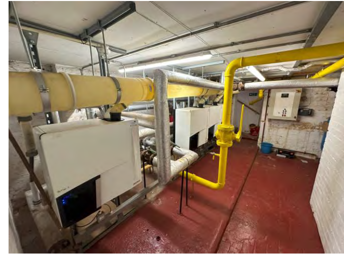
Basement – Boiler Room
