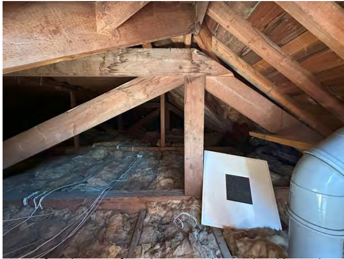
Roof void. Signs of condensation observed and limited insulation at ceiling joist level
