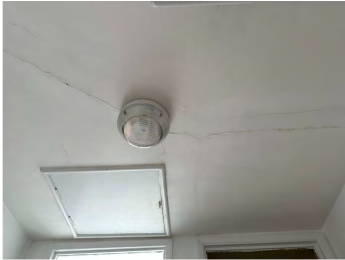
Male WC (110) – Cracking observed around loft hatch
