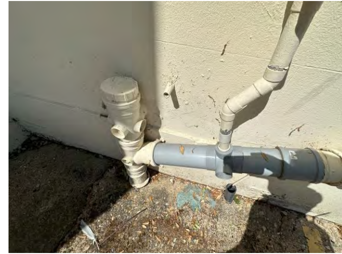
uPVC Above ground drainage pipework painted
