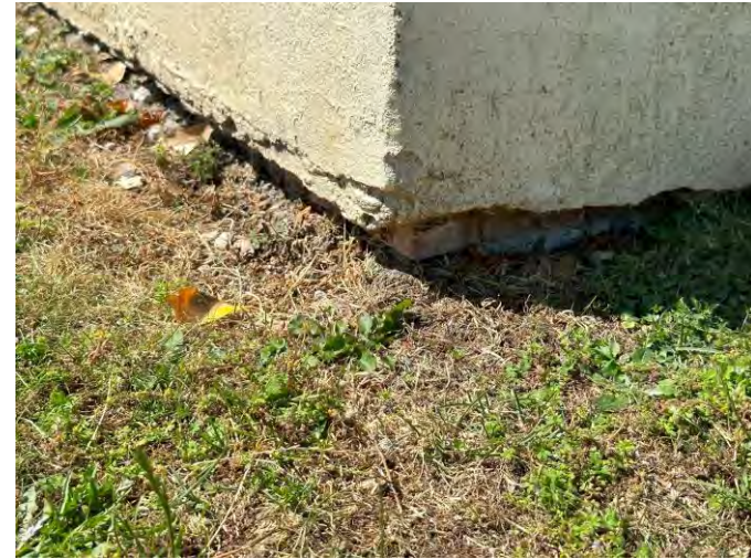
North east elevation – Undulations observed to render at base of plinth on the northern elevation.
