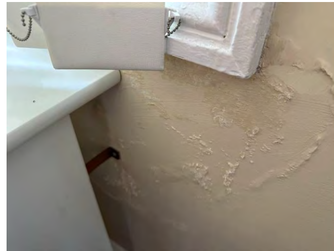
Mayors Parlour (104) - Flaking and blistering to external west facing walls.
