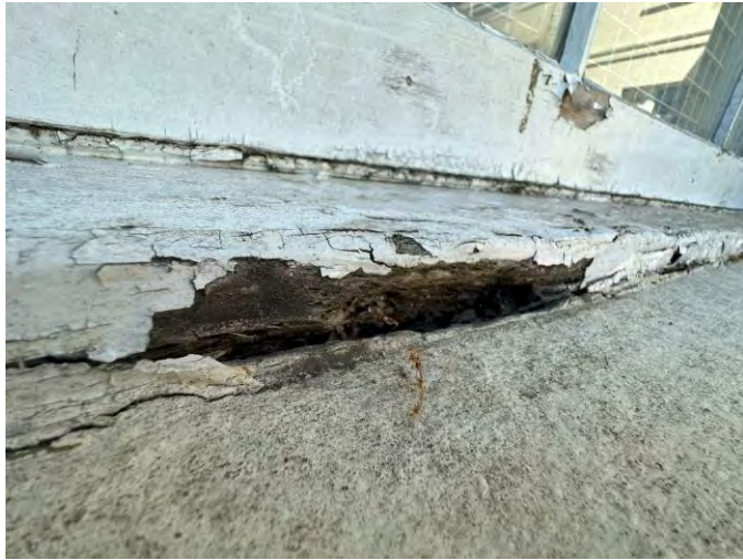
Advanced decay to rear timber window cills
